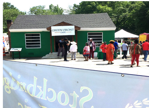
The Green Front Café is currently under renovation. Photo credit: Melissa Jest/HPD
