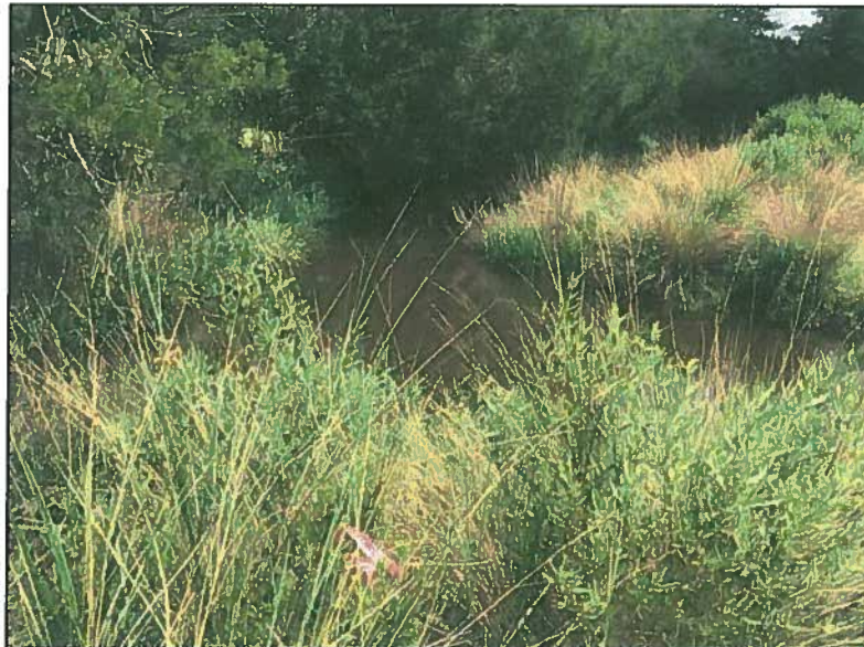
Existing culvert under Sea Island Road, to be extended for sidewalk installation.
