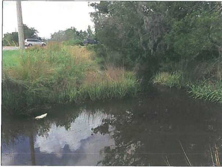
Existing culvert under Sea Island Road, to be extended for sidewalk installation.
