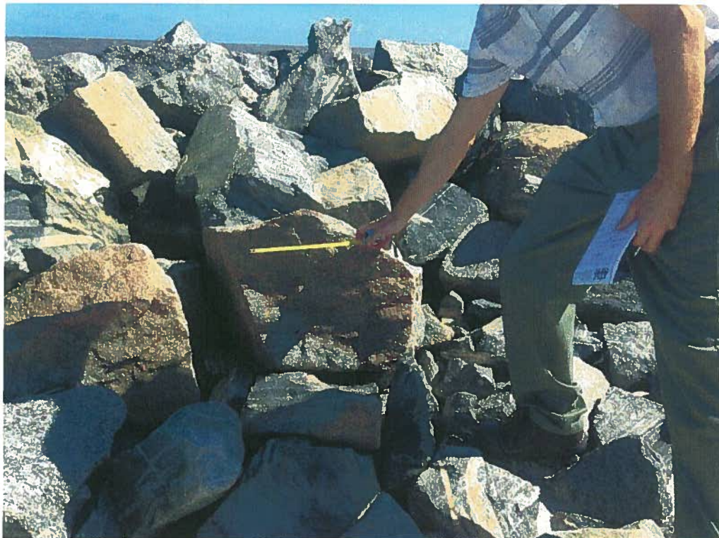
Typical rock size distribution in a fair condition section of the revetment
