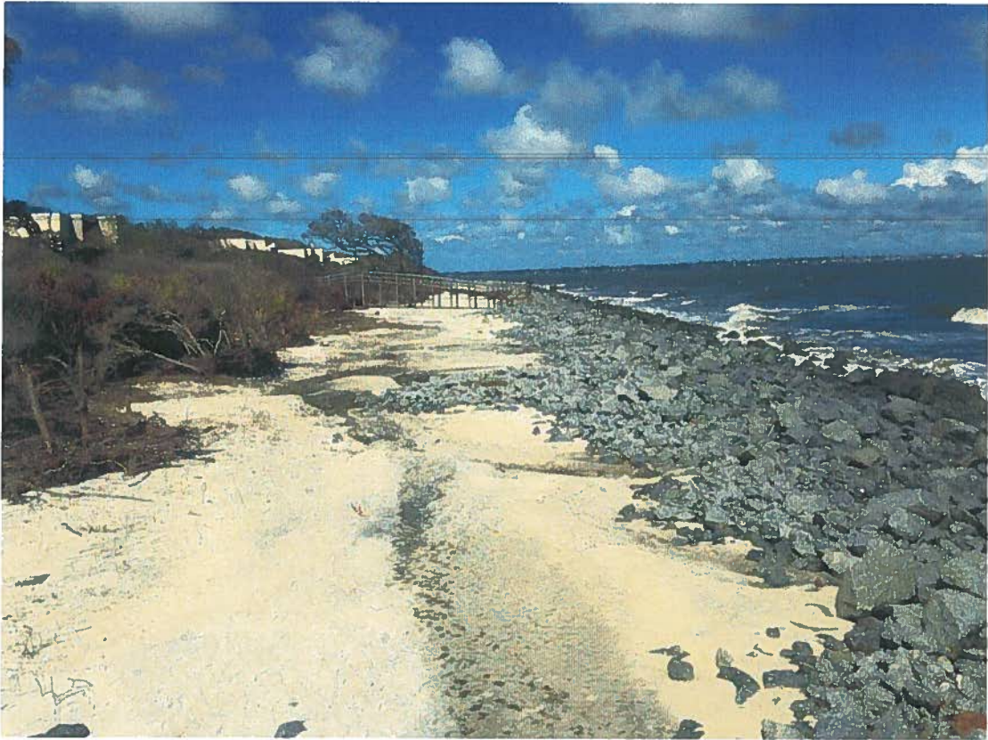
Typical revetment damage, scattered small stone, and dune/upland erosion post-Irma, Villas by the Sea (10/13/17)
