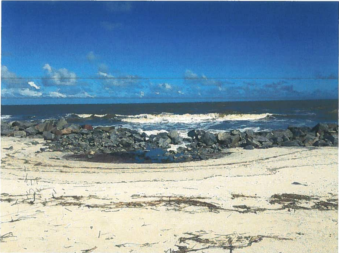
Locally damaged revetment crest section with ponding landward of the structure (10/13/17). Water level ~ MHW (+2.6 NAVD88) at the time of the photo.
