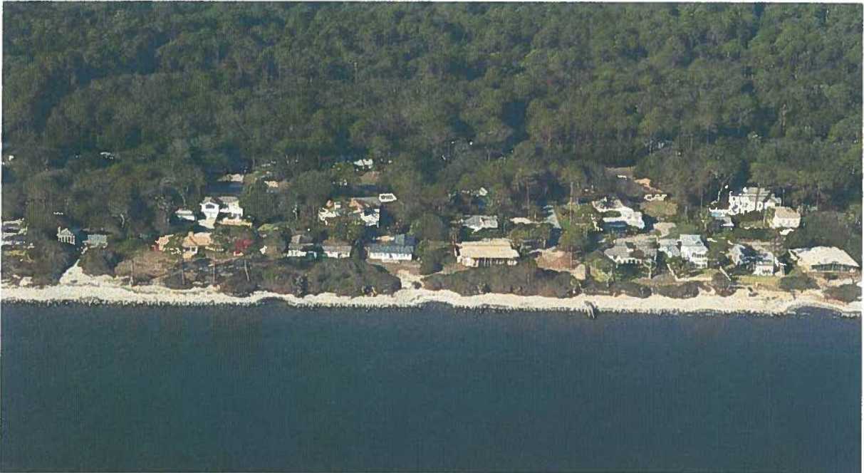
Albright Lane area (Zone D) photo during a "king" tide, showing penetration of water landward of revetment where the crest is low (post-hurricane Matthew photo)
