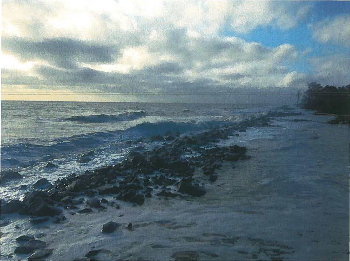
Wave action overtopping a low section of existing revetment during a “king” tide (10/19/17). Note large percentage of small stone.
